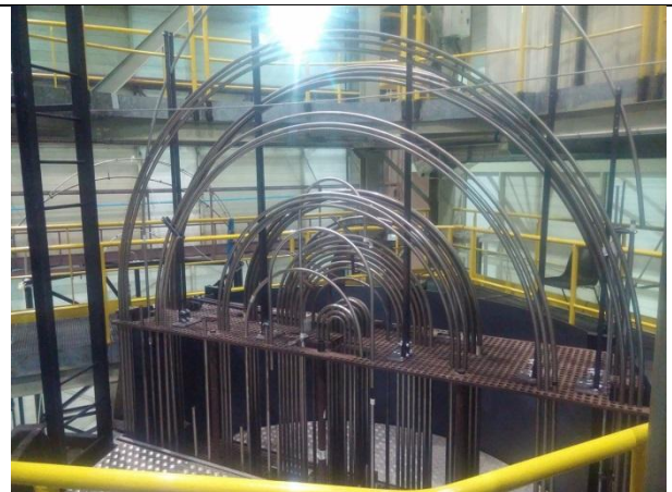
FIGURE 7: STEAM GENERATORS U-TUBES
