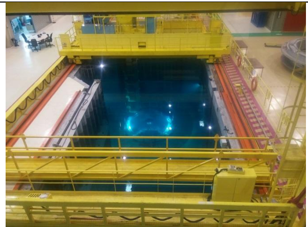
FIGURE 5: FUEL LOADING MACHINE
